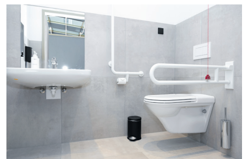
General barrier-free WC
